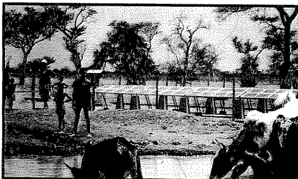
Solarex Photo Solarex array powers water pumping system in Senegal
